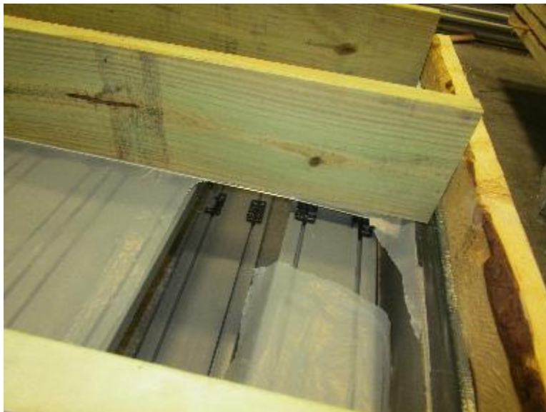
Photo No. 2 Typical Failure (Plastic Clip Releasing from Aluminum Rail)
